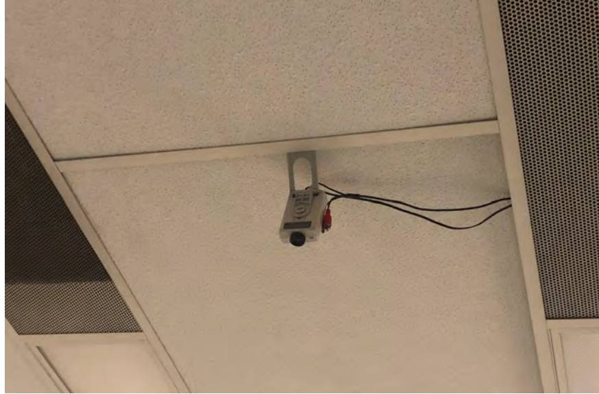
Figure 6: NTSC Camera Hanging from the Ceiling
